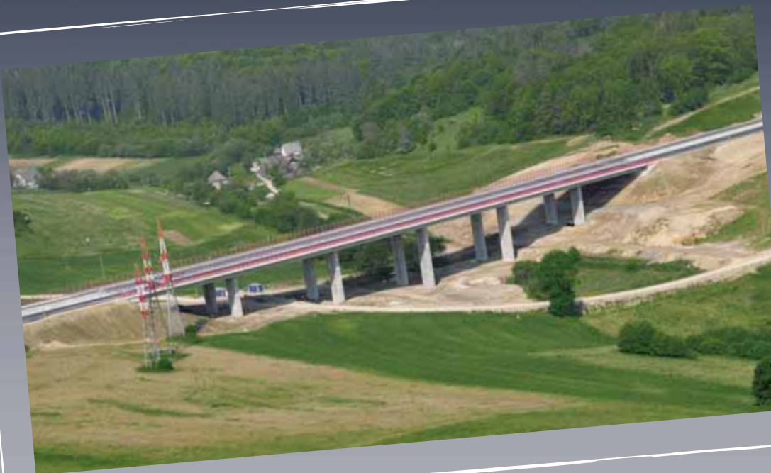
Most 203 - zhotovený technológiou výsuvnej skruže Bridge - Structure 203 - constructed by the incremental launching method
